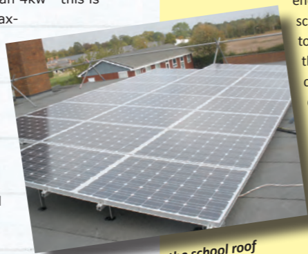
Solar panels on the school roof
